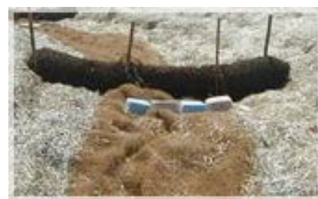
Floc Logs are highly effective for removal of particulates therefore, much smaller detention basins were required
