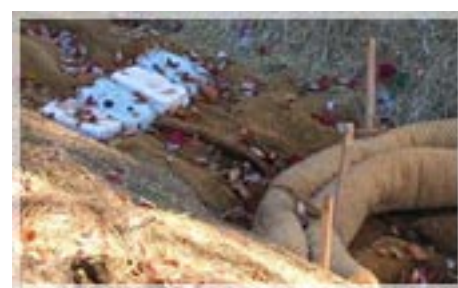
Terra-Tubes and Floc logs are secured with wooden stakes to withstand 1500 gal/min of water flow
