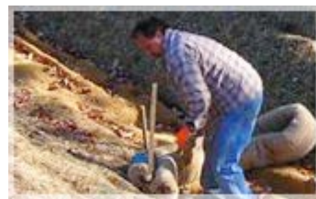
A combination of Floc Logs and Terra-Tubes are carefully positioned in the swale
