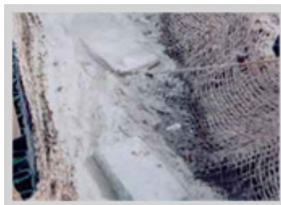
Reaction of the turbid water with the Floc Logs caused the sediment to bind together and collect on the jute matting.
